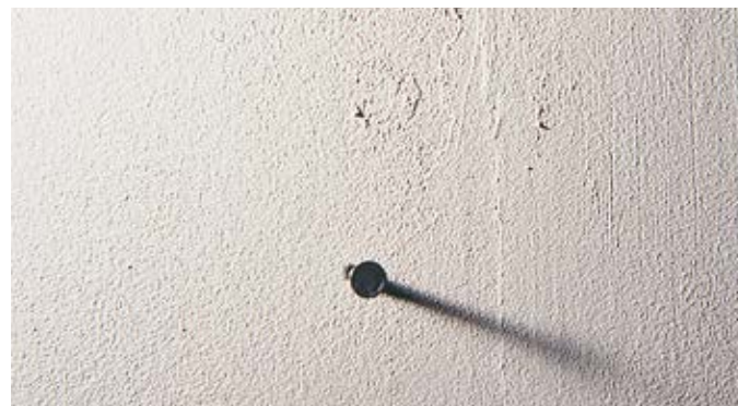
The same plasterboard joint under glancing light
